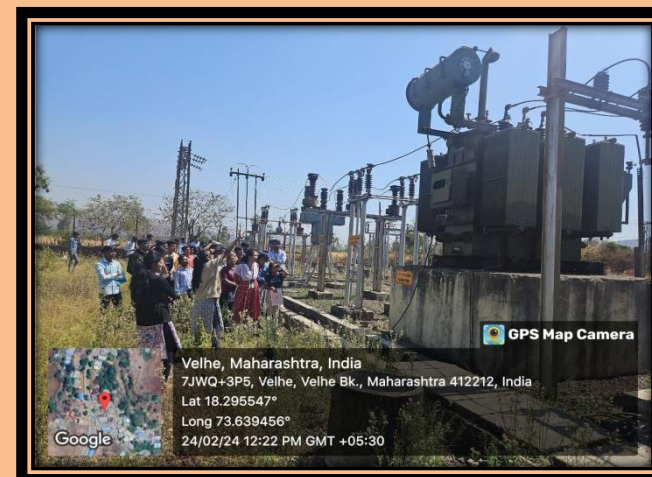
66/22 KV Substation, Pabe
